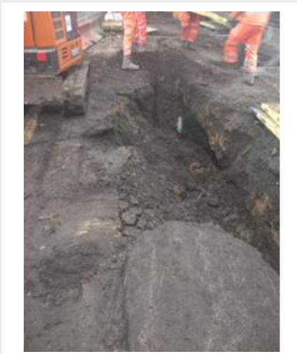
Sidewall failure and make up of ground
